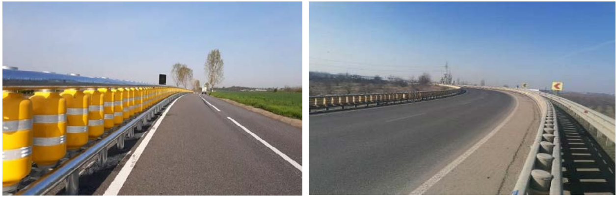
Figure 4. Sections of guardrails on rollers on national roads.
