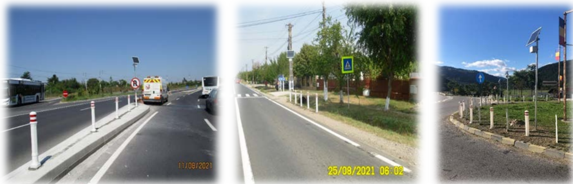
Figure 11. Lighting assemblies mounted on hazardous sectors.
